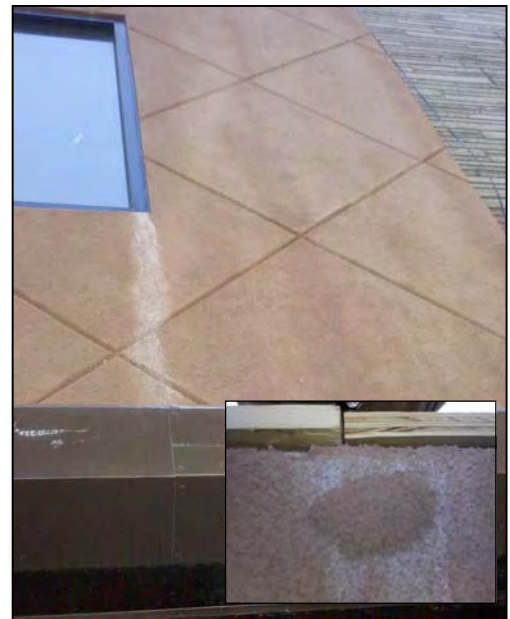
This finish was installed in cooler weather and left unprotected. Inset photo – efflorescence check showing original color
