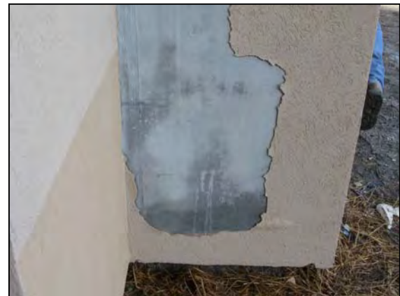
Blistering and wash off caused by cool weather application...and a leaking downspout
