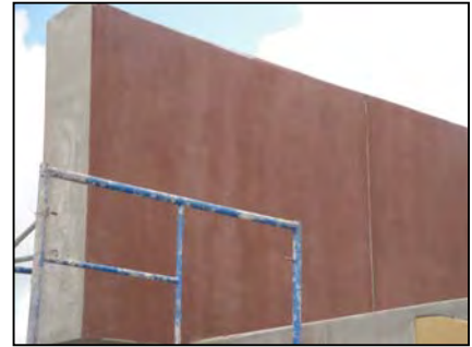
Uncapped wall lead to a streaky appearance on this dark color
