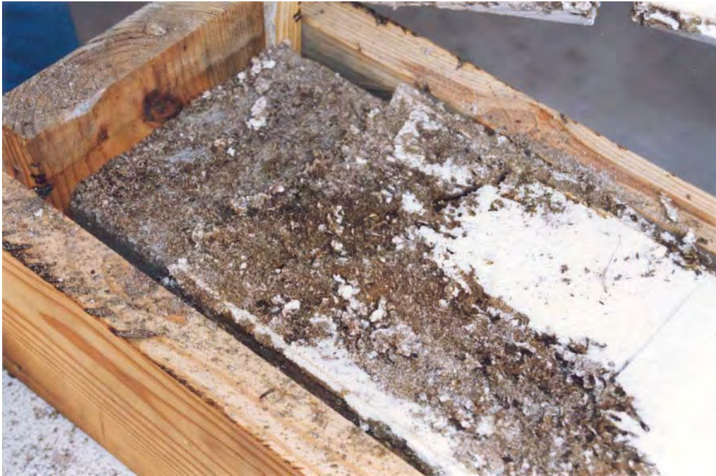
#45 TEST FIXTURE - Close-up shows extensive termite damage.
