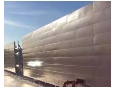
Example of oil canning a.k.a. buckling or surface variation on a metal building
