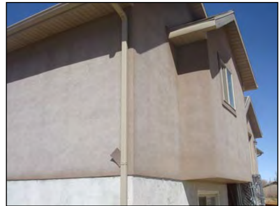
This home had "fading finish". It's not fading, it's efflorescence. Original color at downspout.
