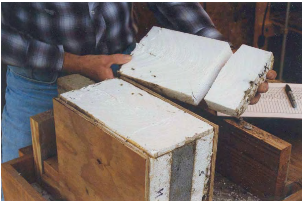
#64 TEST FIXTURE - Close-up shows slight termite damage.
